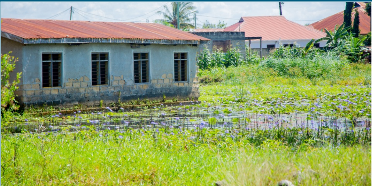
Figure 8: House located in the flood prone area in Tanga
